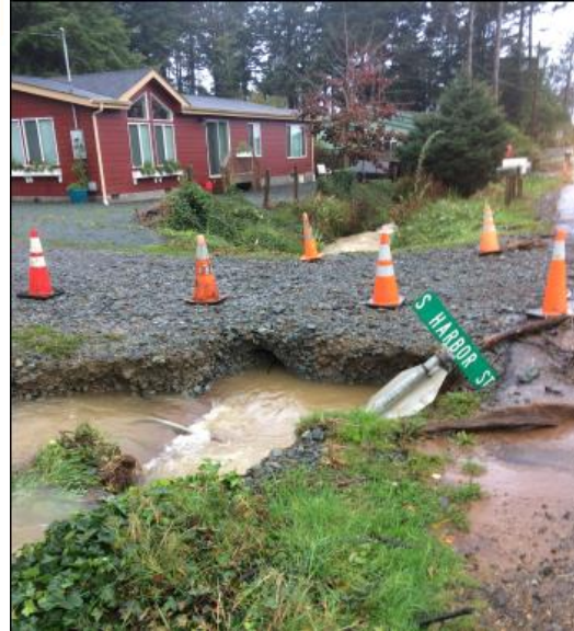
Typhoon Songda Culvert wash out October 2016
