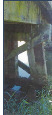
Wyss Bridge – Rotten Column
