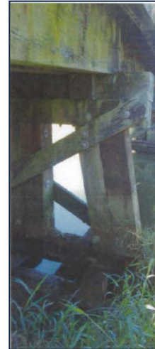
Wyss Bridge – Rotten Column
