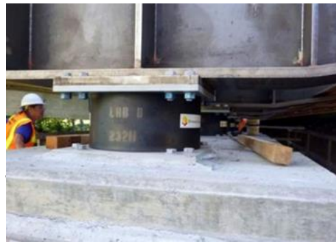
Lommen Bridge - Dynamic isolation bearings minimize damage during earthquakes
